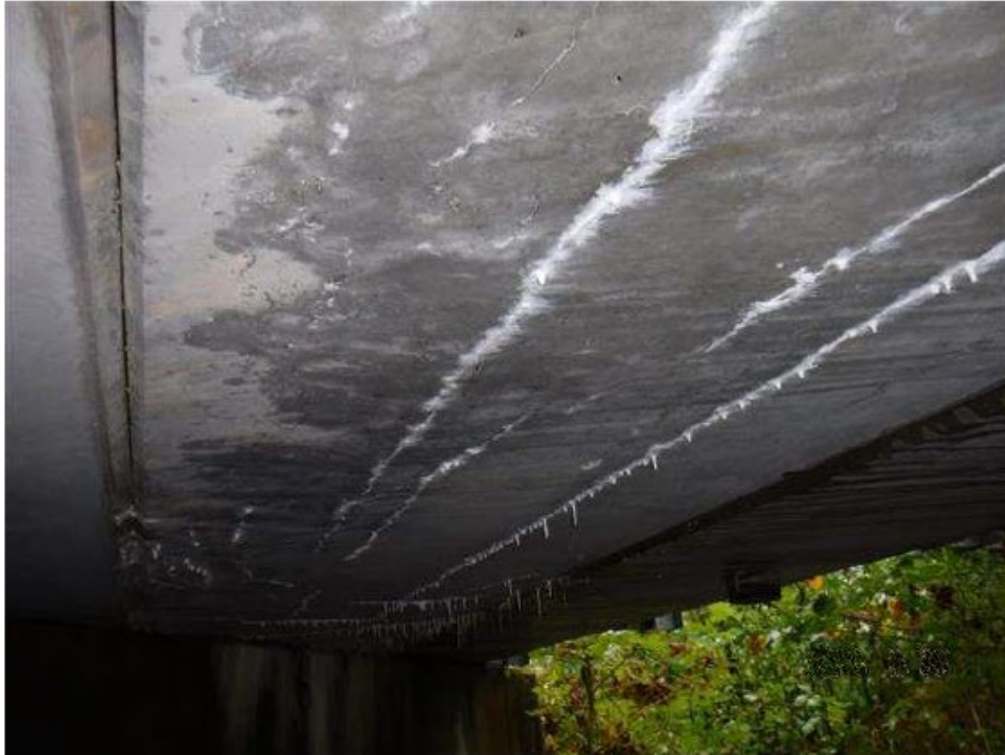
Cracks in Beam 2A
