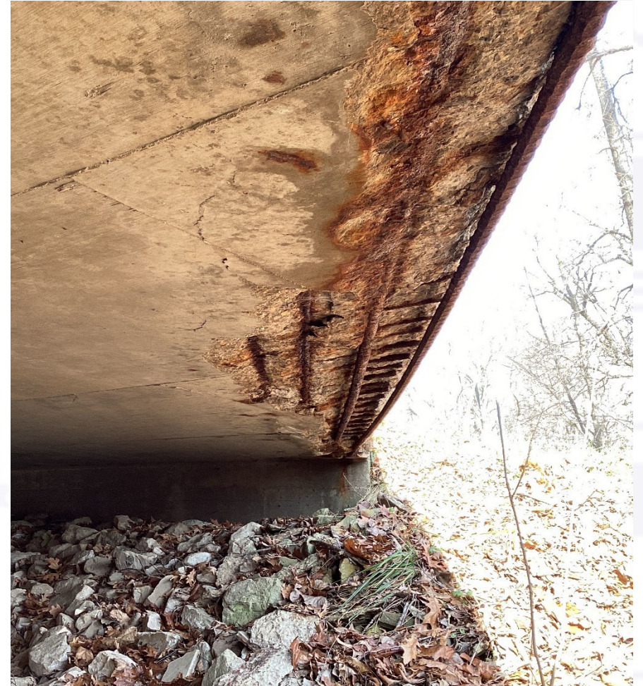
Exposed Steel with Heavy Corrosion along the West Coping of Span A Superstructure
