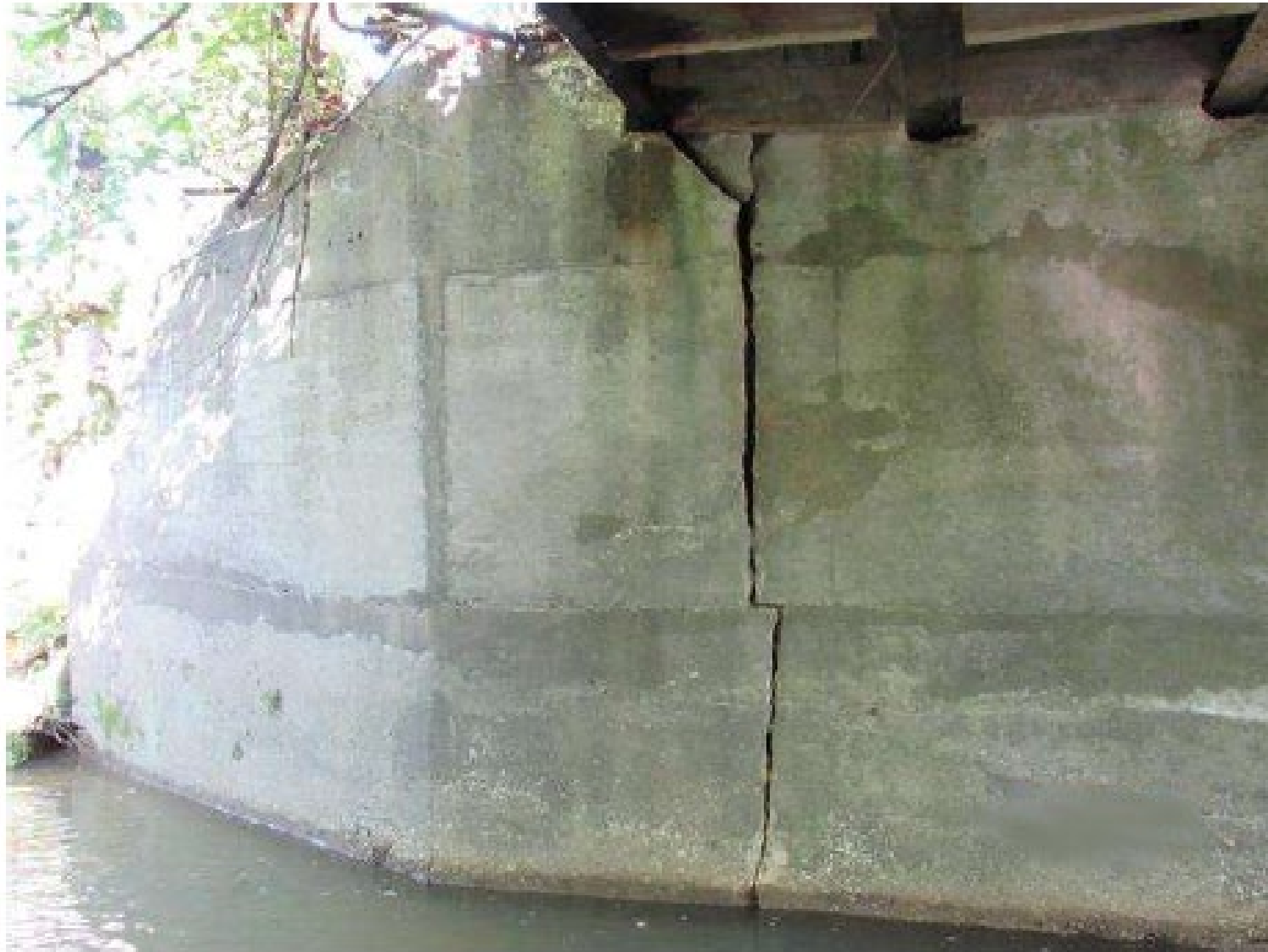
Crack at Northwest Corner
