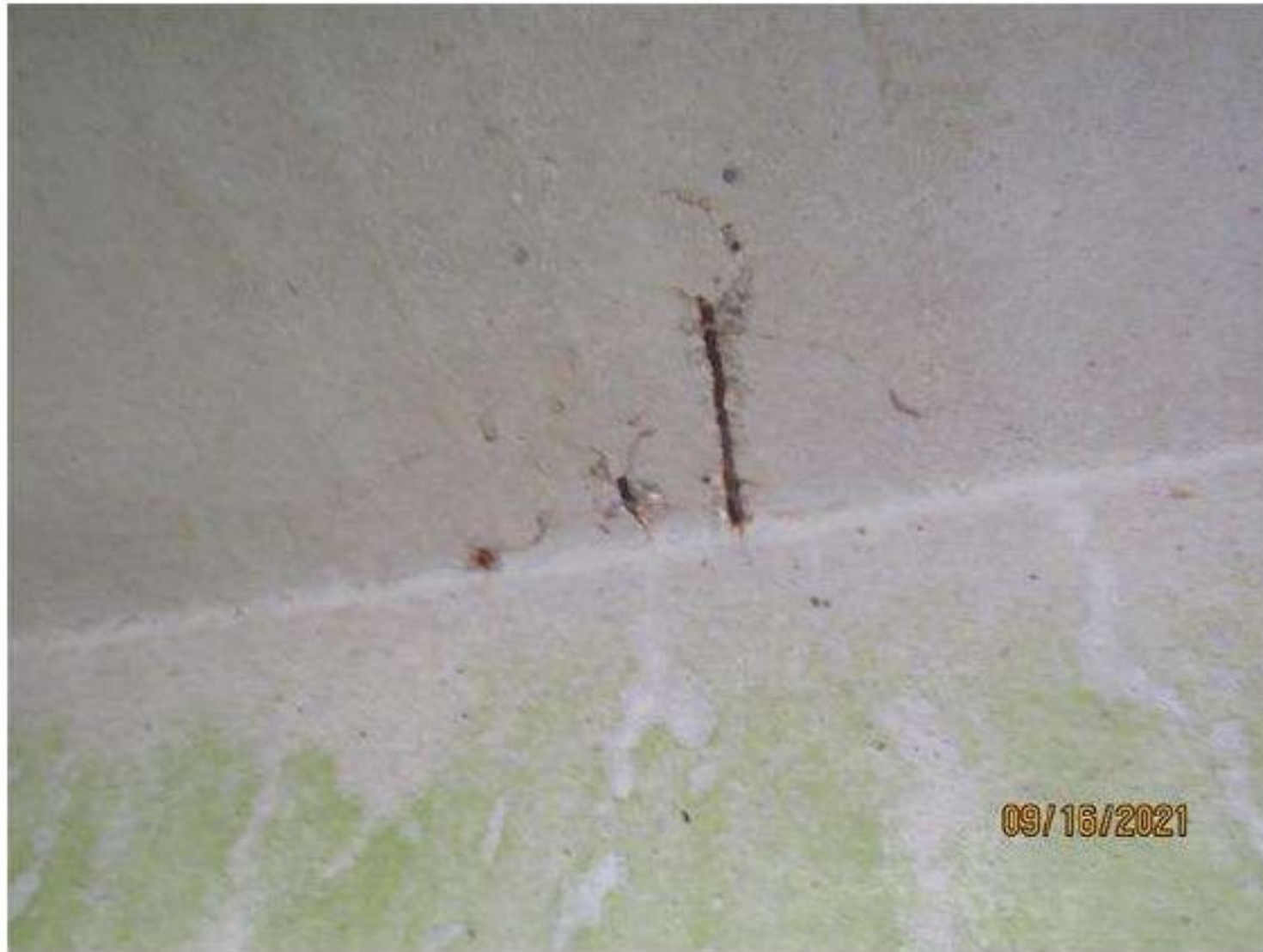
Spalls in Top of Beam (Centerline of Structure)
